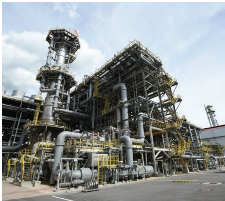
Close-up view of the Petronas LNG Complex near the town of Bintulu
