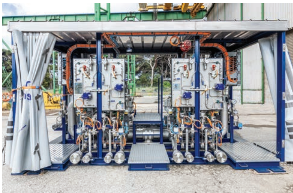
A skid's system's control panel plus connections
