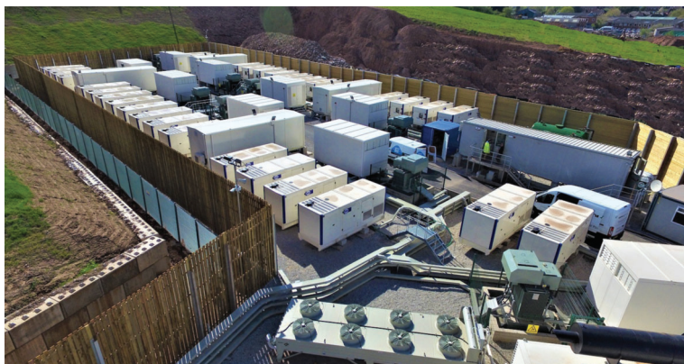
Gresham battery storage units
