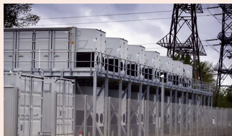
UK's first, 50 MW grid-scale battery storage
