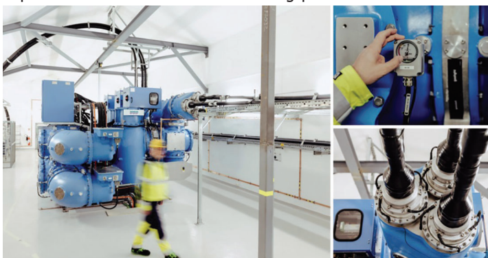
SF6-free switchgear at the Koengen substation in Bergen, Norway
