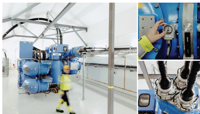
SF6-free switchgear at the Koengen substation in Bergen, Norway
