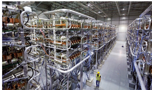
View into Siemens SVC Plus
