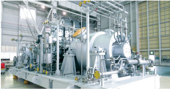
MHI-built ammonia syngas train
