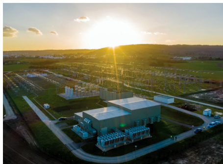
View of a STATCOM system in Kriftel, Hesse, installed on behalf of Amprion
