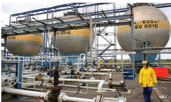
GenCell site with ammonia tanks in Israel
