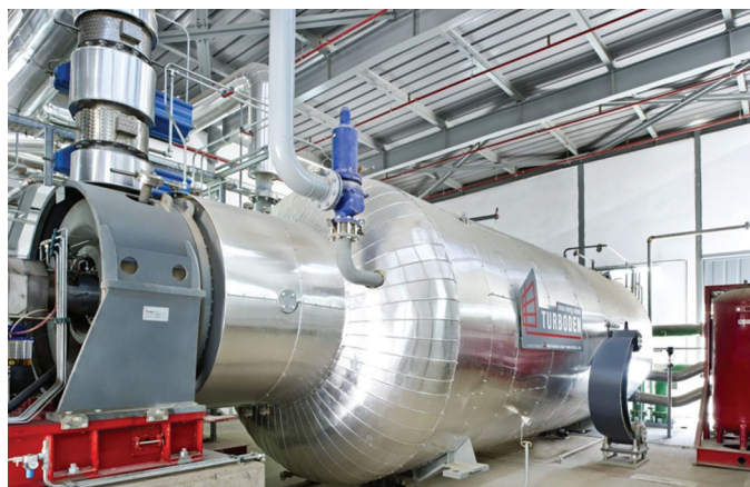
Installation of a Turboden ORC system
