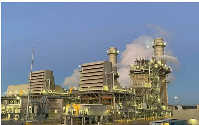
Montgomery County Power Station in Willis, Texas
