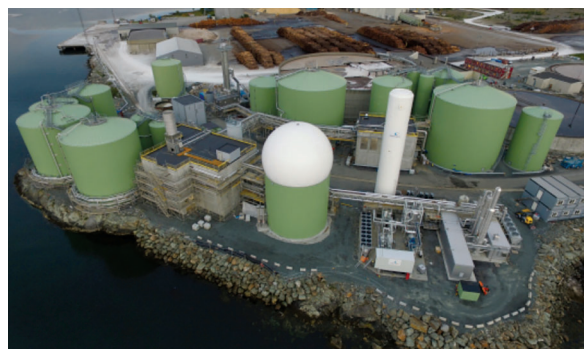
Biogas upgrading and liquefaction unit at Skogen LNG terminal
