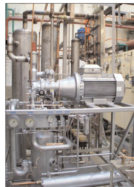
Figure 1: Small-scale LNG pilot plant
