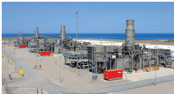
Part of Medgaz process facilities for Algeria-Spain pipeline
