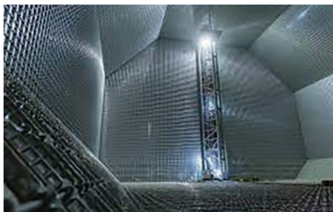
GTT containment tank
