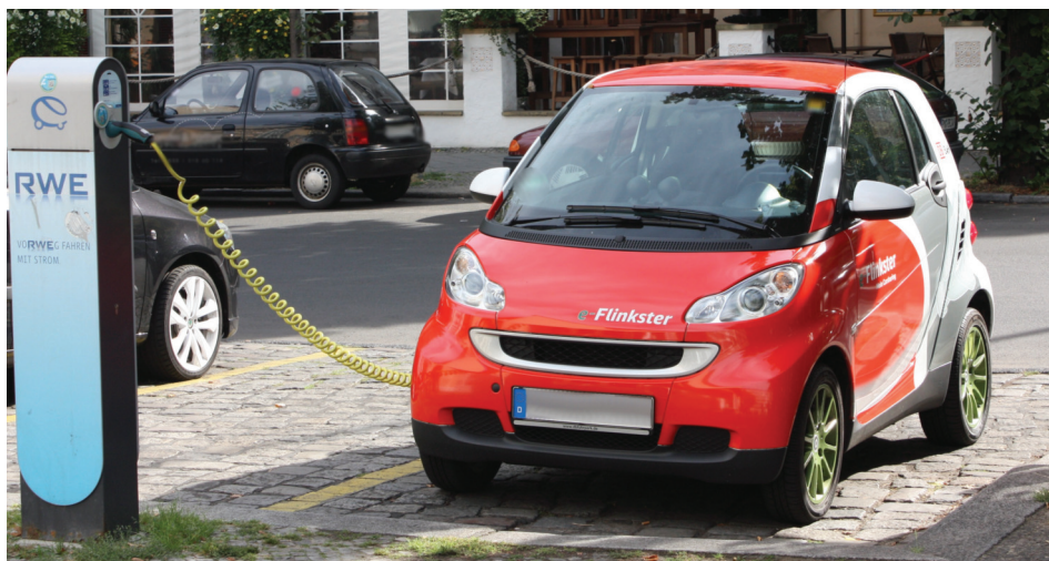
RWE e-vehicle charging station in Germany
