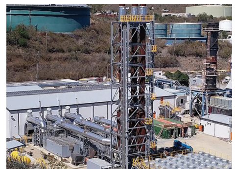
Randolph Harley power plant site, where the hybrid unit and storage will be installed
