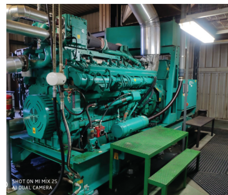
Cummins' QSK60G generator at TROIL Vegas Altas plant
