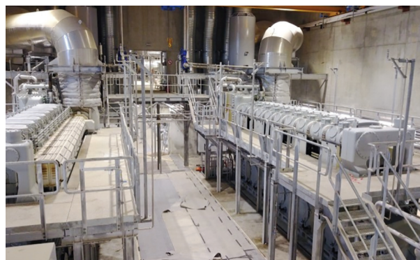
Four MAN engines will add 37 MW to the Sund power station
