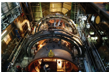
GT26 turbine installed at JFE's Chiba power plant in Japan
