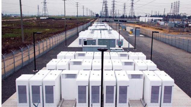
80MW PowerPack substation in Mira Loma, California.
