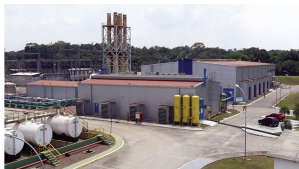
Cristiano Rocha power plant in Manaus
