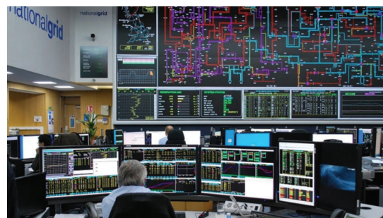
View into the control room of National Grid UK
