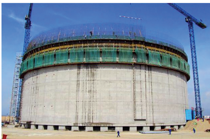
China is continuing to ramp up its import terminals
