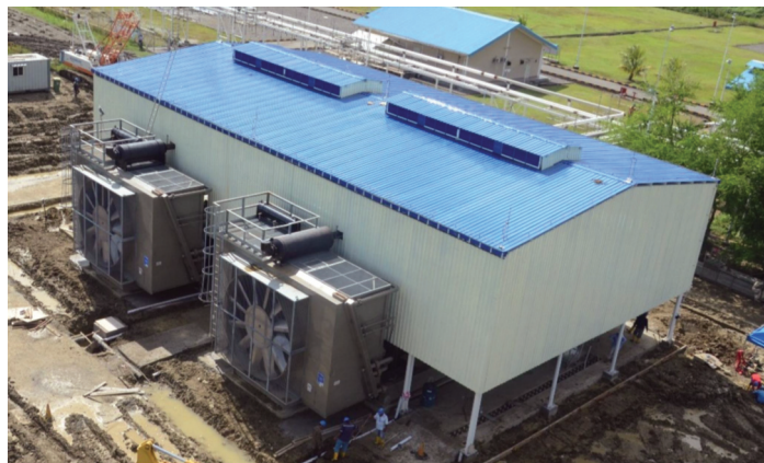
Compressors at Kampung Baru will boost Sengkang plant
