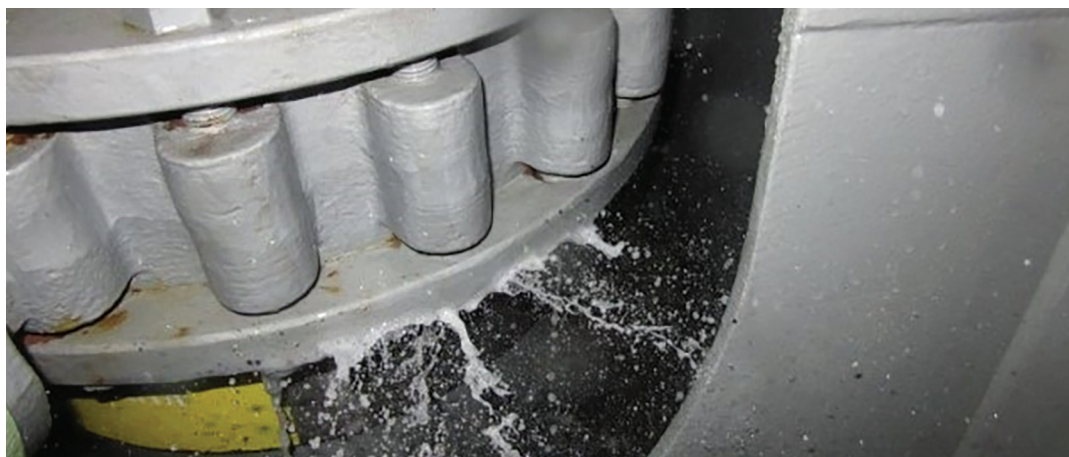
Water ingress as a result of a corroded scrubber pipe
