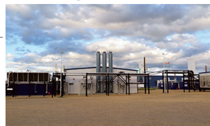
LNGo system installed for Altagas in Dawson Creek, BC
