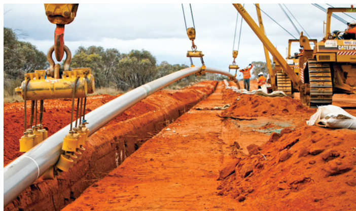
Chinese company will offload Western Australian pipelines
