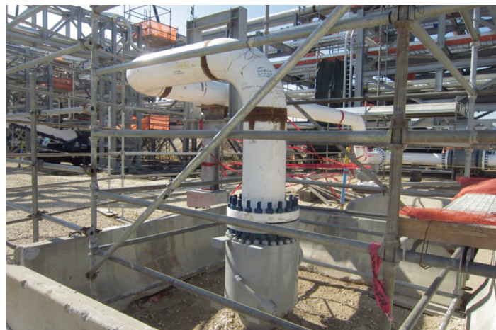
Feed-gas tie-in at the Elba Island plant near Savannah
