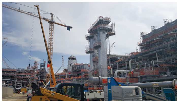
Pre-treatment area of latest liquefaction plant
