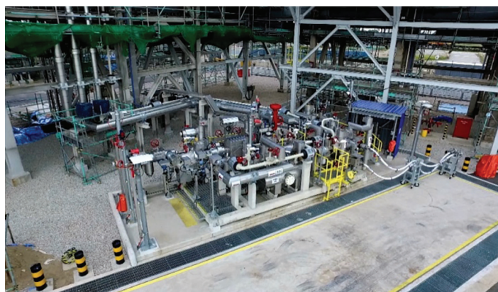
Aerial view of Singapore's first LNG truck loading facility
