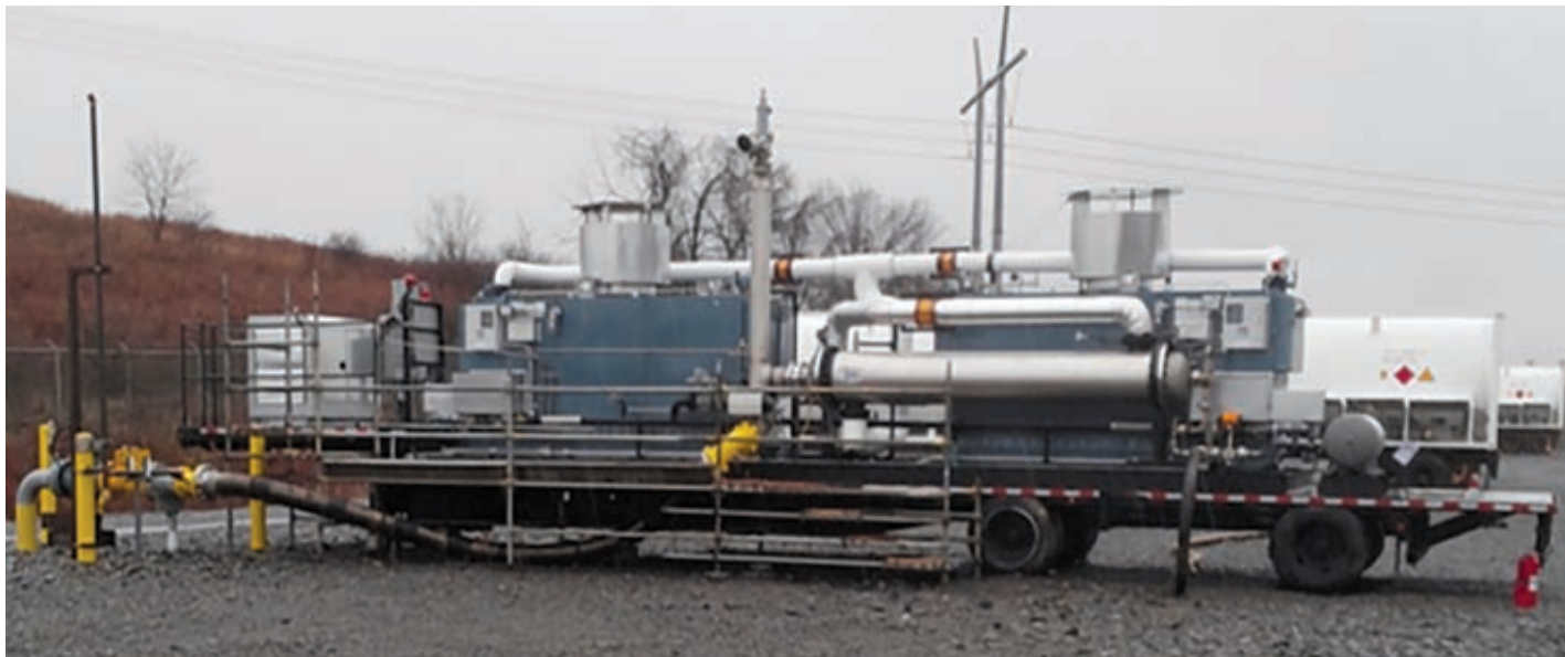
Hot water LNG vaporizers also supplied to Longview plant
