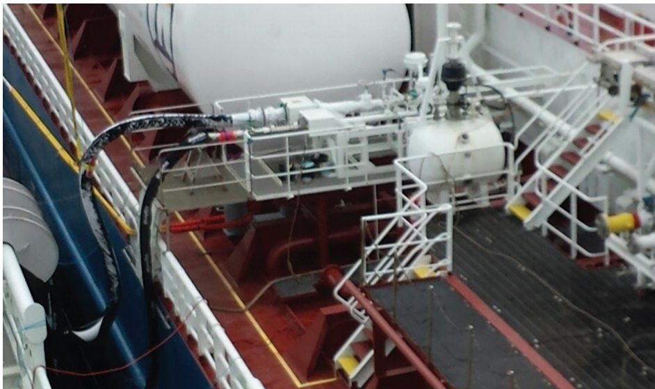
The cryogenic hose connection can clearly be seen.
