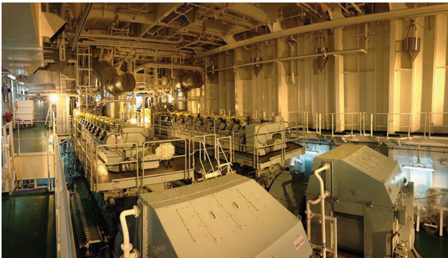
Panorama of the engine room aboard the Velikiy Novgorod featuring a diesel-electric, dual-fuel propulsion system consisting of 2 × MAN 8L51/60DF and 2 × MAN 9L51/60DF engines.
