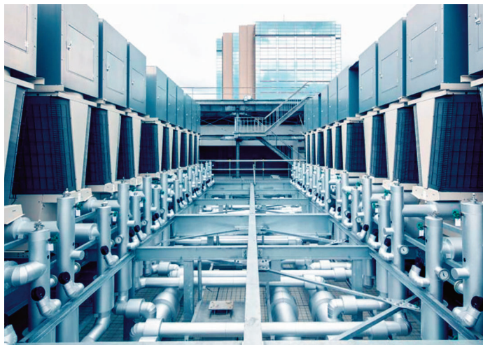
Tokyo Fuchu Data Center
