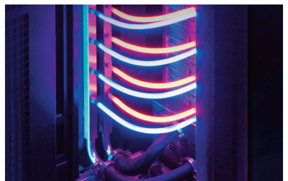
Close-up of KAYTUS liquid cooling
