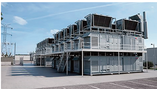
Rolls Royce's modular gas engine power plants
