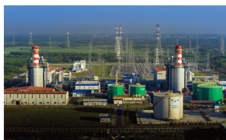
PV Power's Nhon Trach 3&4 LNG-fuelled plants
