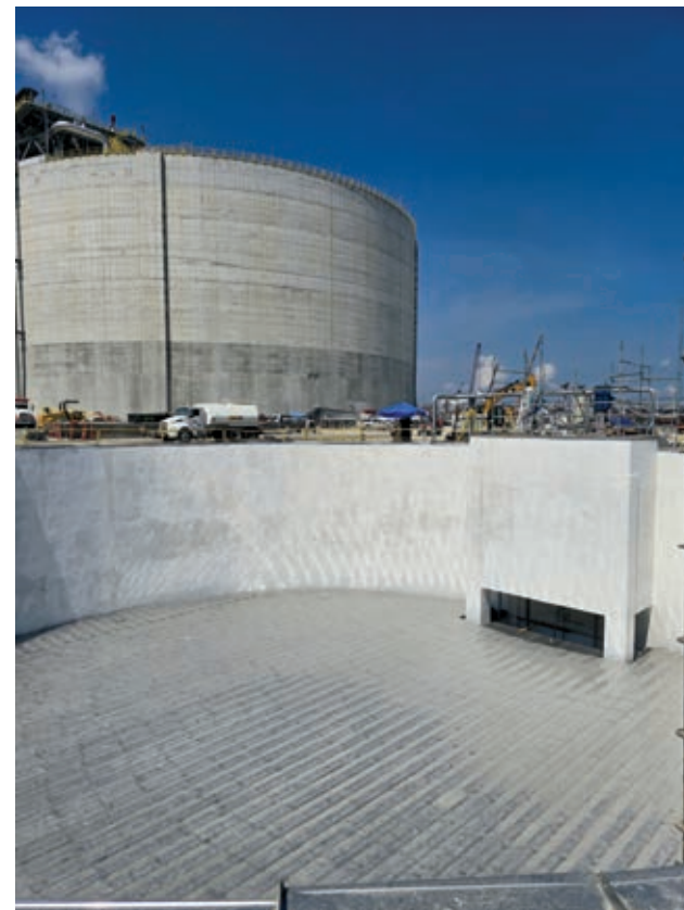
PFS Installed at an LNG facility
