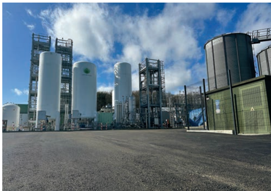
Sublime Energie demonstrator system
