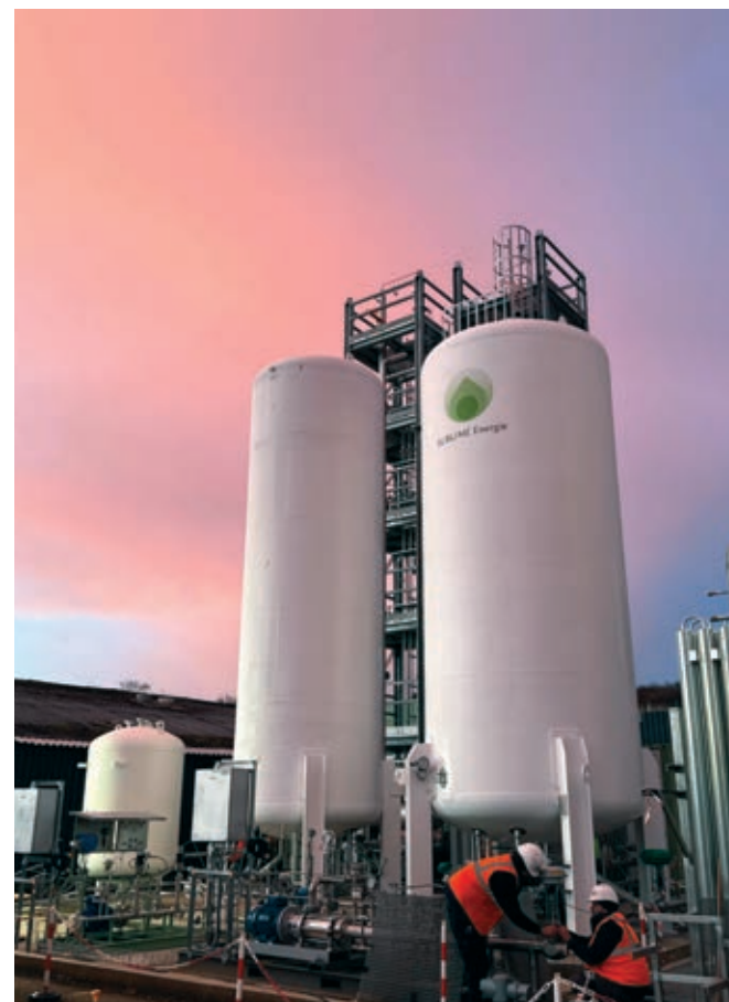
Storage tanks on site
