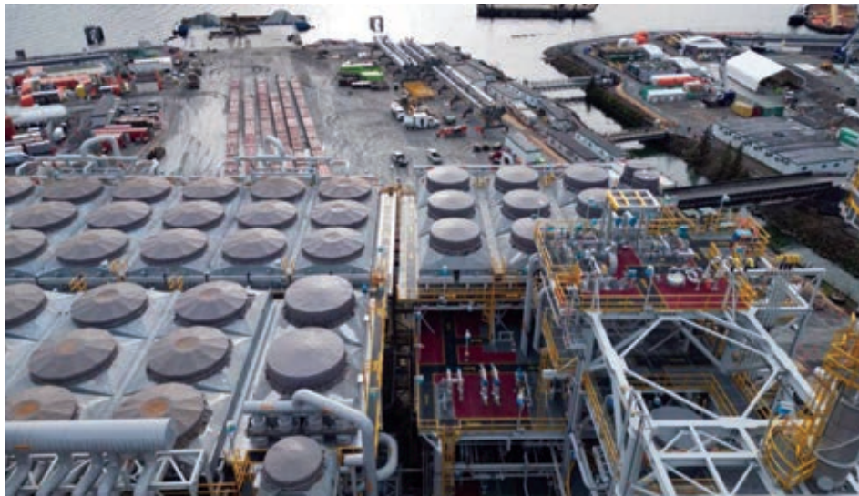
Woodfibre LNG module with air-cooled heat exchange system clearly visible
