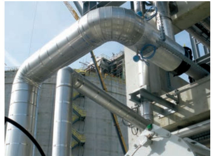
FOAMGLAS® cellular glass fitted on an LNG terminal
