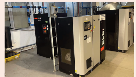
Close-up of EGL compressor
