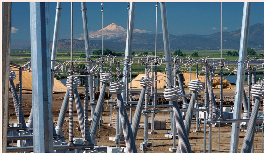
Avangrid substation Klamath
