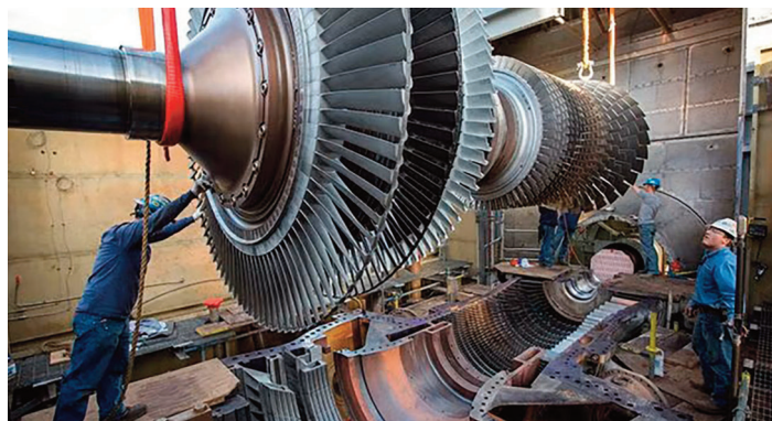
View into PSM gas turbine repair facility in Jupiter, Florida
