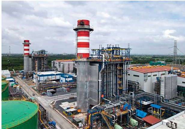
PV Power's Nhon Trach power plant
