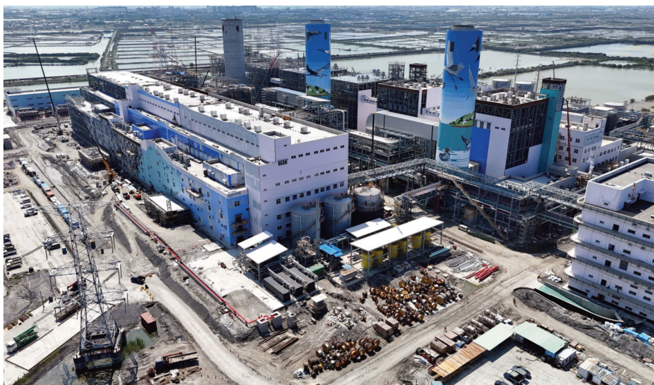
Taipower's Hsinta power plant
