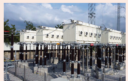
PG&E smart wires substation
