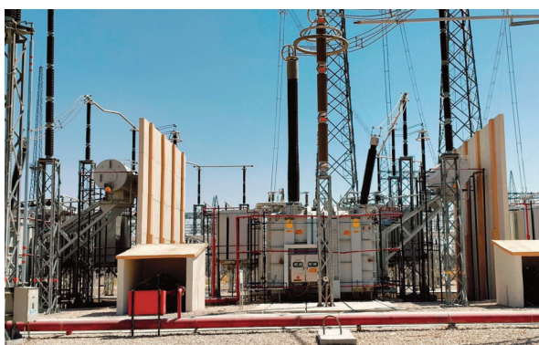
GE high-voltage transformer in action
