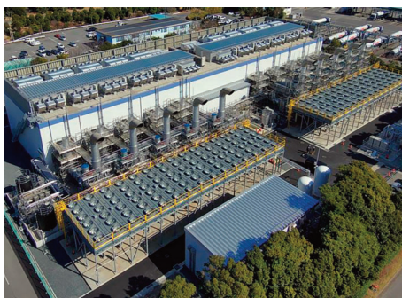
Sodegaura power plant
