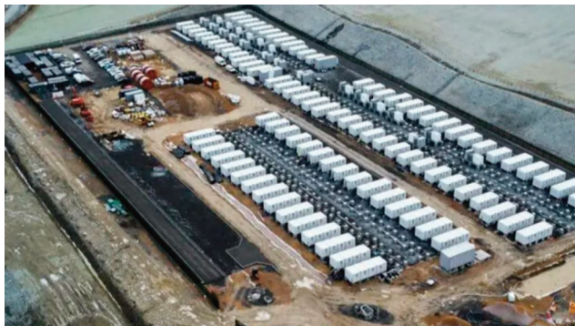
Very large battery energy storage in Blackhillock
